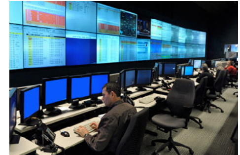
Bell National Operations Centre.
