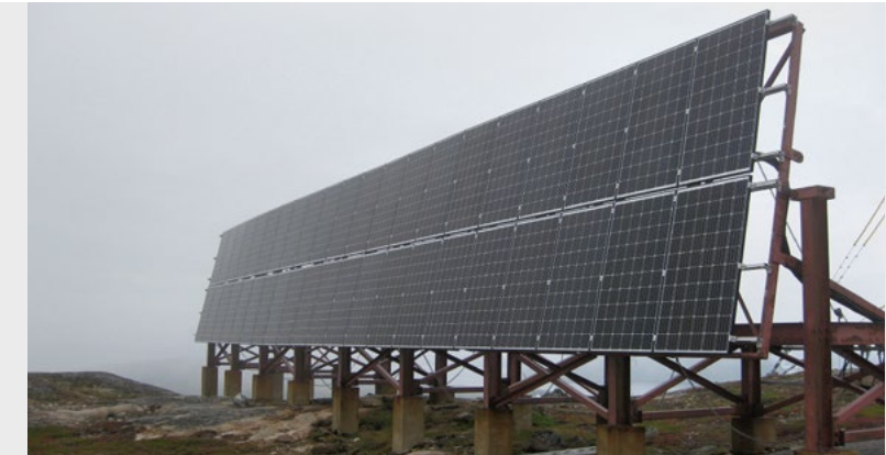
HYBRID SOLAR/DIESEL CYCLE CHARGE SITE
