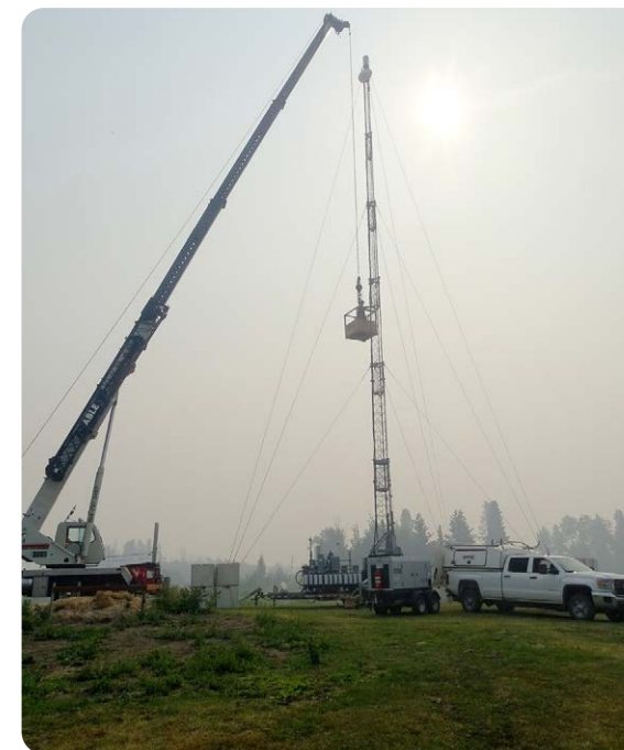
In response to wildfires in Manitoba during the summer of 2021, Bell MTS teams from Network, Field Services, Customer Operations, Real Estate and Emergency Management worked together to keep Bell sites and equipment online.
