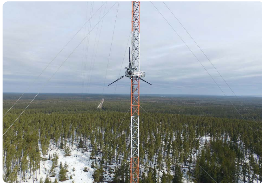
In Ontario, our wind and solar power technologies installed at 12 remote cell sites generated approximately 50,000 kWh of renewable energy every year.
